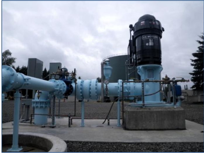
Rockwood Water PUD Well
